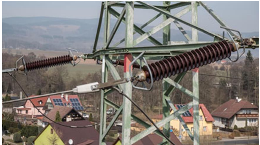
Joint on the high voltage distribution line. The place where a problem may occur, i.e. origination of transient resistance with consequent overheating.
